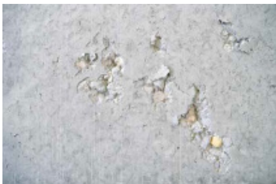
Fig. 4.7 Tearing off at the concrete surface
