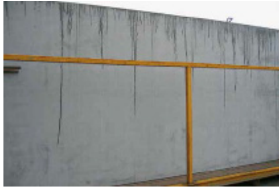
Fig. 5.4 Unprotected storage: water marks
